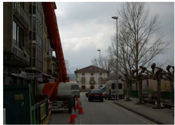
Calle renovada, luminarias FHS_{inst} = 0\%
